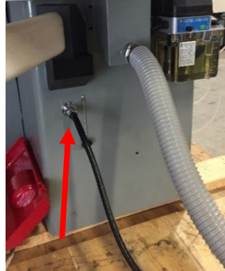
Filter Pump Line/plug
