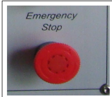
Dwg. 2.3 Emergency Stop
